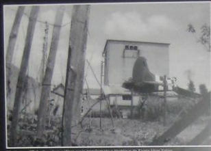
Dangerous working of a man going on to the Electrical Transformer.
